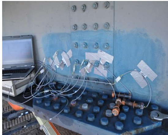
Figure 5.13: Loosened bolts connected with the terminal
