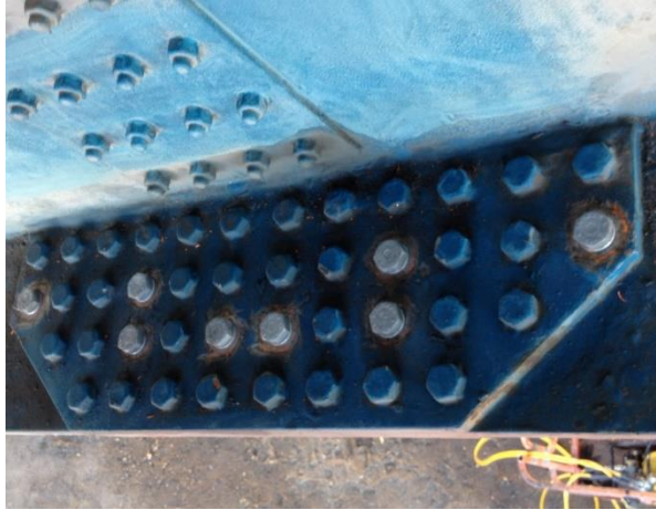
Figure 5.18: One side of the connection after the measurements
