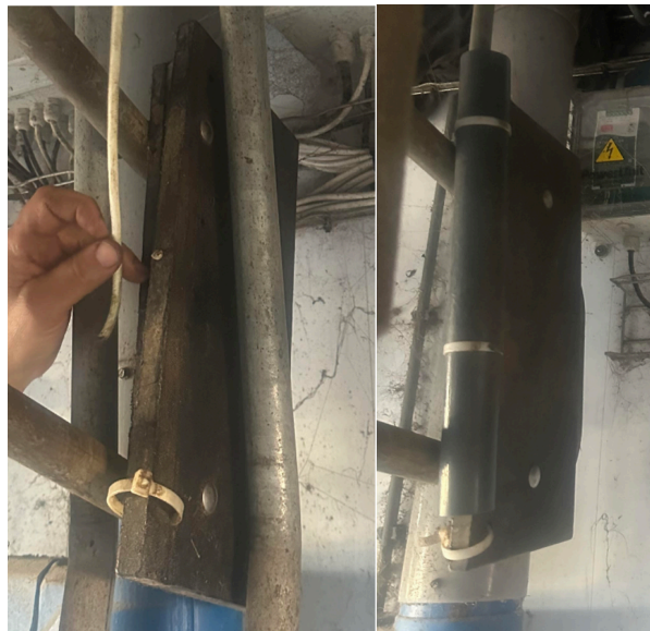
Figure 13: A broken and temporarily repaired competitor antenna cable with PVC covering
