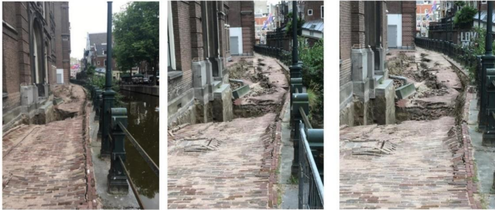
Figure 6.7, Photographs taken during the collapse of the Grimburgwal. The quay wall is progressively leaning towards the canal side. Behind and on top of the quay, settlements and sinkholes are present.
