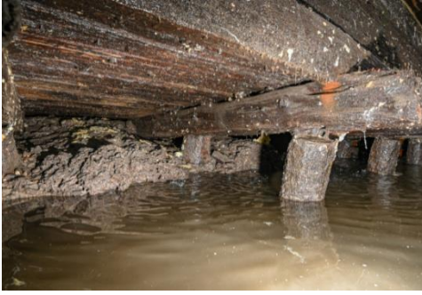
Figure 5.9, Photograph of pile-headstock connections below a historic quay wall in Amsterdam (Maarschalkerweerd, 2022).
