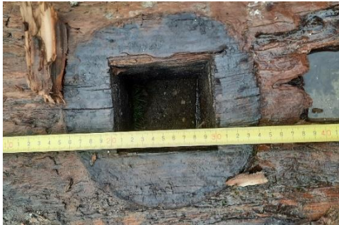
Figure 6.4, Headstock extracted from collapsed Grimburgwal with pin hole and pile imprint visible (Korff et al., 2021).
