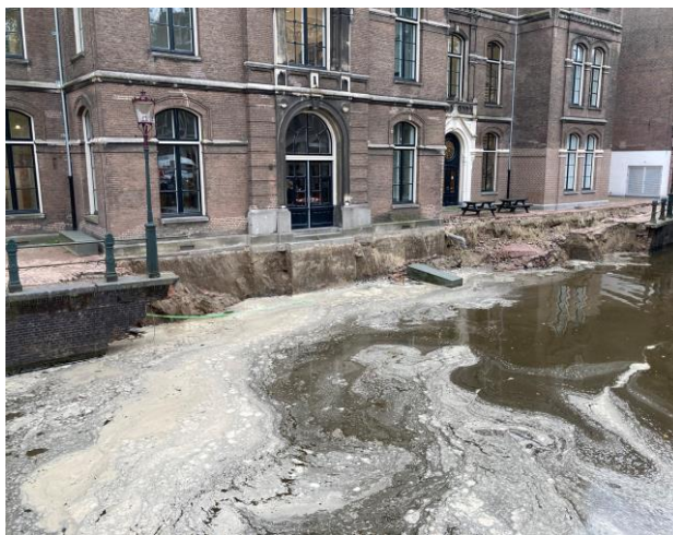
Figure 6.1, Grimburgwal directly after failure. Building in the background is the University of Amsterdam (building GB2). Left side of quay is ‘East’ and right side of quay is ‘West’. Photograph: Hugo Logtenberg, 1 September 2020.
