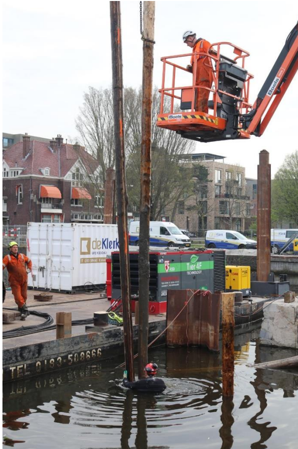
Figure 4.28, Temporary new timber pile (right) is removed and directly replaced with fibre-optic-installed pile (left).
