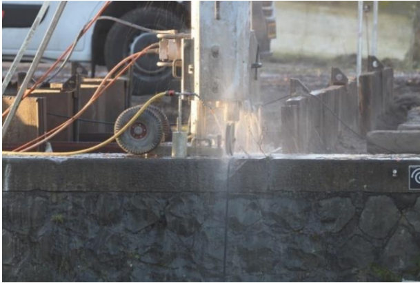
Figure 5.19A, Cutting through the gravity wall and timber foundation with a bandsaw to decouple segment from sides.
