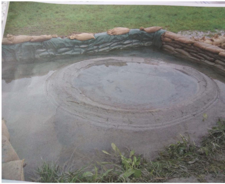
(a) Frequently reactivating sand boil near Guardia Ferrarese along the Po river, Italy [Martínez et al., 2020].
