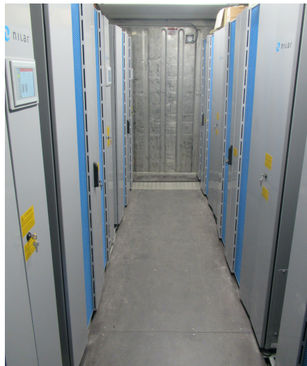
Figure 3.6: Installed NiMH battery racks in container
