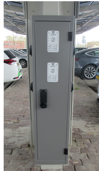
Figure 3.7: Installed EV charging station
