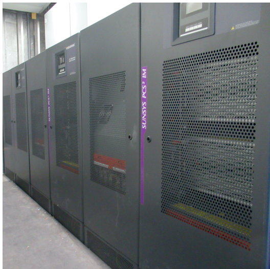
Figure 3.5: Installed battery inverter in container
