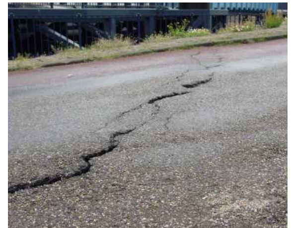
cracks in a road due to jet scour
