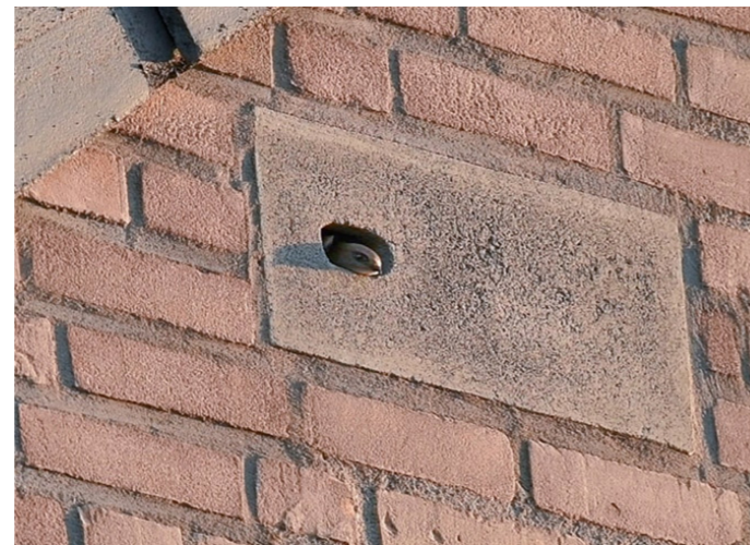
Use of birdbox in facade-Stedenbouw.nl
