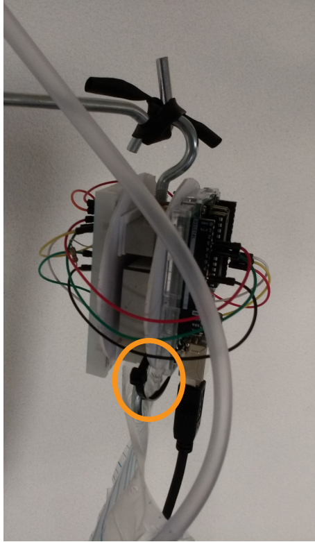
Figure 27.2: Tie rib that disturbs the measurements
