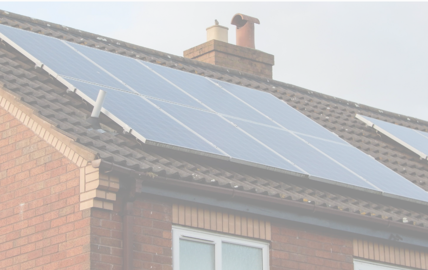
Figure 71: Rooftop with several solar panels installed
