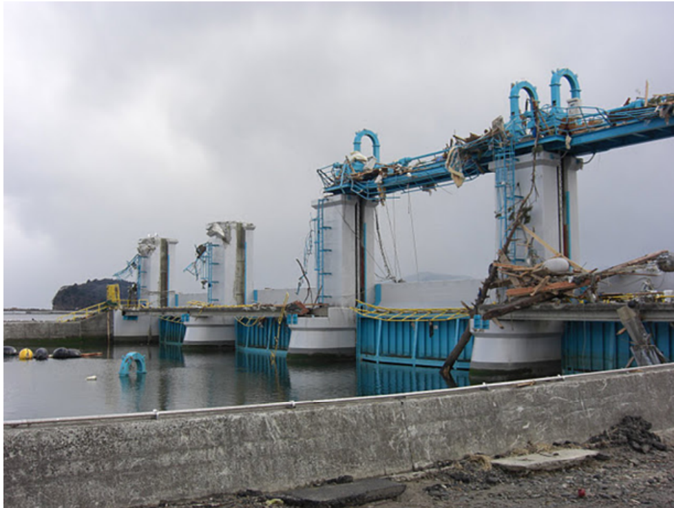
Figure: Damaged floodgate at Minamisanriku
