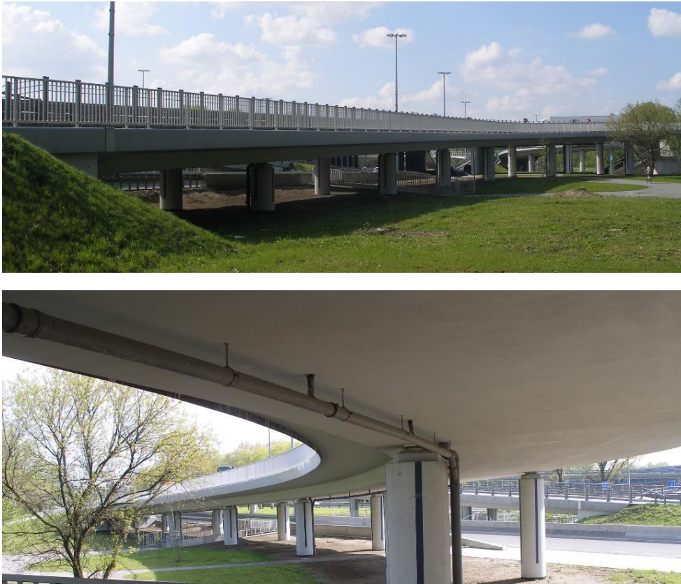
Figure 1 – Bridge views after applying anti-corrosion protection and putting into service: on top : from the support side No 1; bottom : from the support side No 8 (support numbering is also presented at Figure 3).
