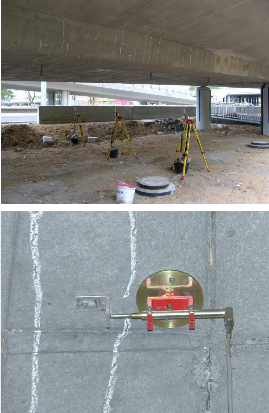
Figure 5 – Preparation of the bridge for the tests: on top : span 2-3 visible inductive sensors to measure the vertical displacements and cracks marked on the structure; bottom : close-up view of inductive sensor to measure the crack width (cracks are marked on the structure).
