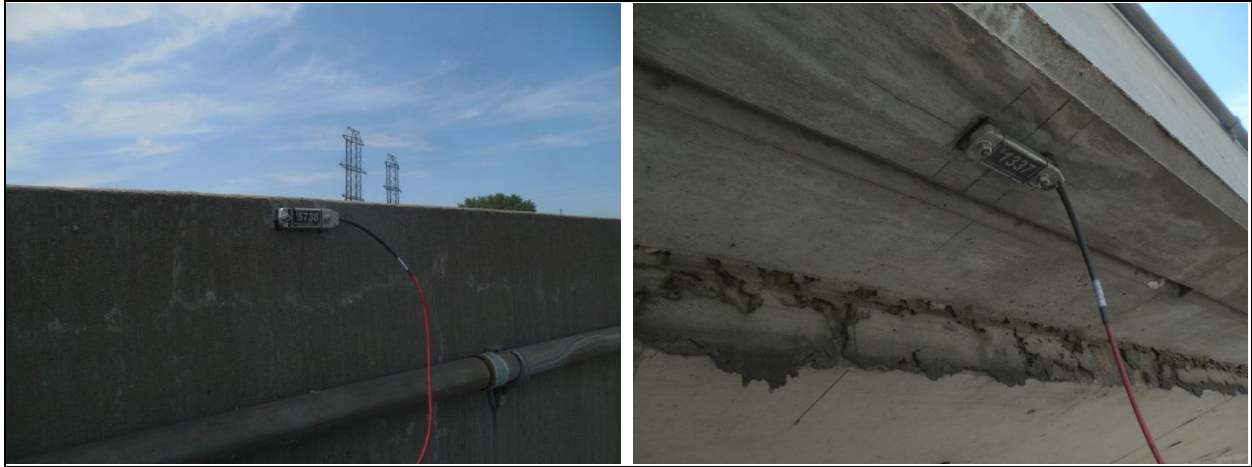
Figure 7 Top and Bottom strain transducers on parapet (typical).
