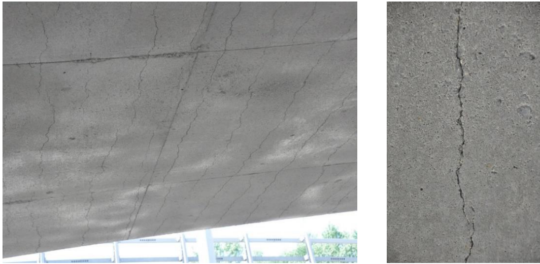
Figure 2 – Views of the cracks on the bottom surface of the slab perpendicular to the span 6-7; right : close-up view of an open crack – crack edge damage is visible.
