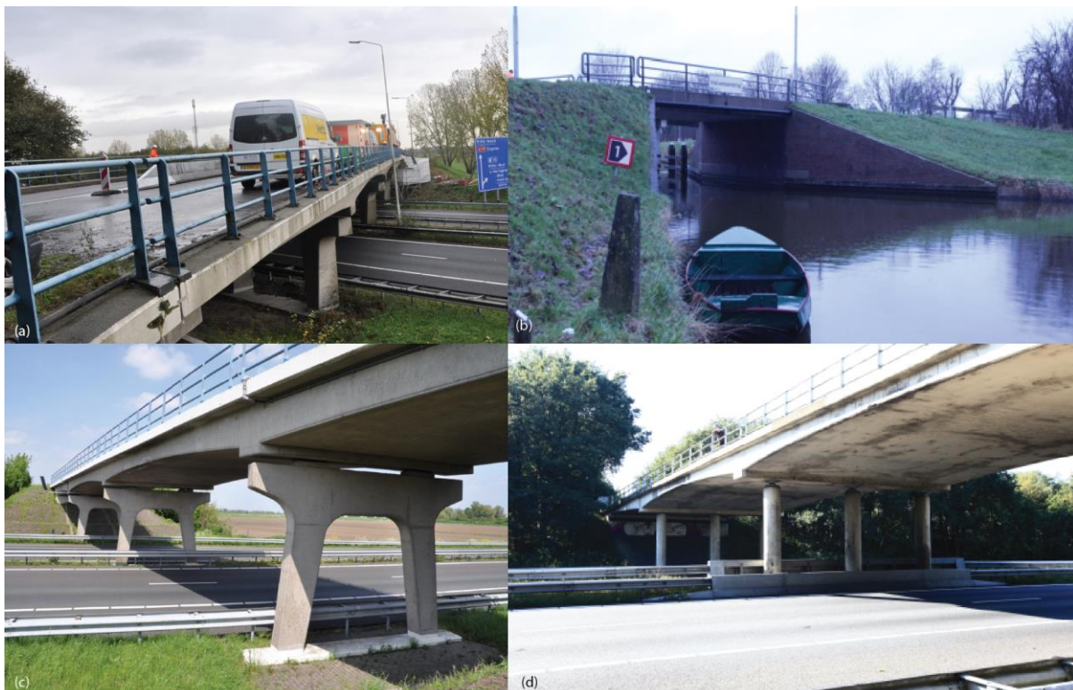
Figure 3 — Overview of bridges tested by Delft University of Technology in proof load testing program: (a) Viaduct Vlijmen Oost; (b) Halvemaans Bridge; (c) Viaduct Zijlweg; (d) Viaduct De Beek.
