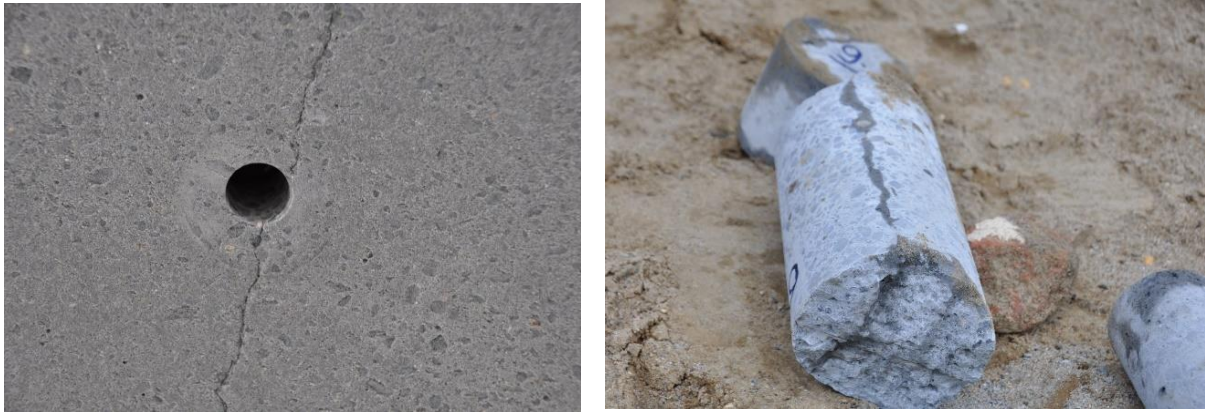
Figure 4 – Cracks width laboratory measurements at concrete borehole: left : crack at drilling place; right : crack at borehole.
