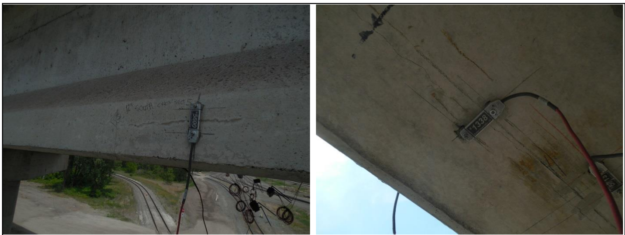
Figure 8 Strain transducers mounted across girder DEF cracks to measure crack movement (typical).
