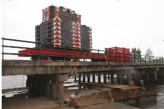
Figure 10 — Use of steel spreader beam, hydraulic jacks, and counterweights in the test on the second span for the Ruytenschildt Bridge.
