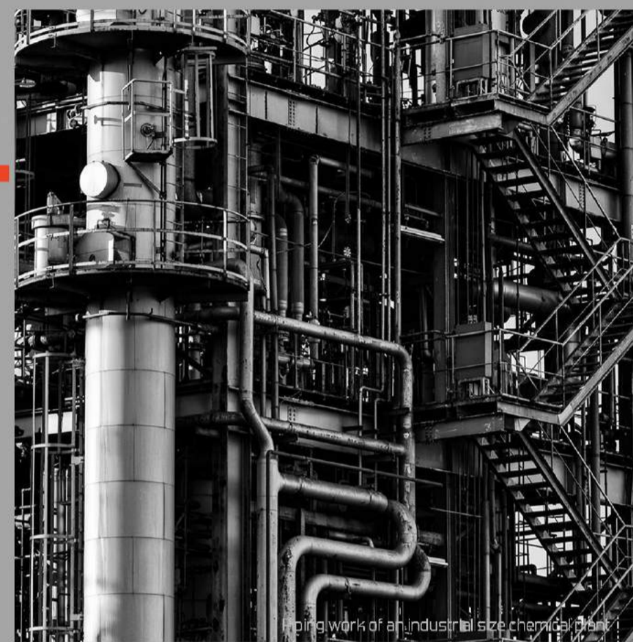
Backbone of an industrial size chemical plant
