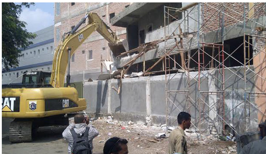
Figure 2. Jakarta City Government forcibly demolished the five-story building in East Jakarta due to land use violation and permit ( http://poskotanews.com/2015/08/12/bangunan-hotel-lima-lantai-dibongkar/ )
