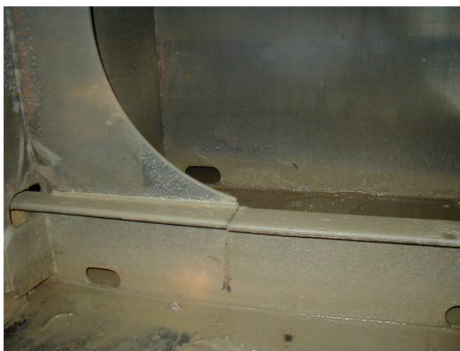
(a) Longitudinal stiffener and bracket with toe crack
