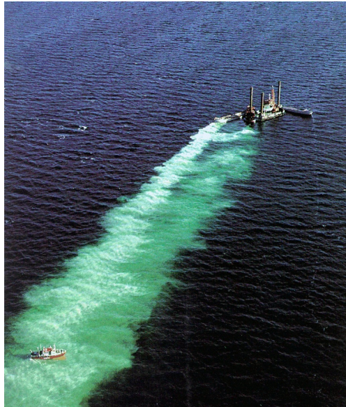
Figure 0-8 The 'Chicago' and 'Coastal Flyer' at work. The sediment plume is clearly visible
