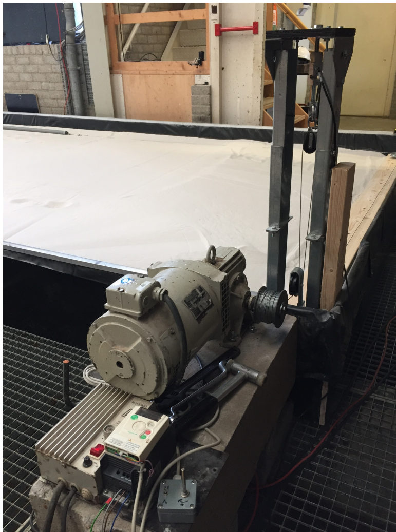
Figure 3.7: Electrical drum winch including frequency drive and measuring tower, located on the sheave beam side of the flume
