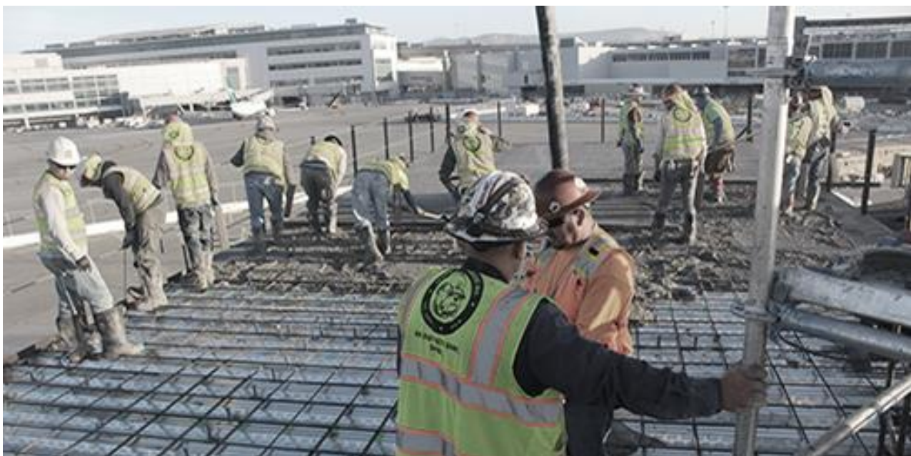
Figure 16: Use of Blue planet aggregates in concrete at San Francisco Airport construction site (Source: https://www.sustainablesv.org )
