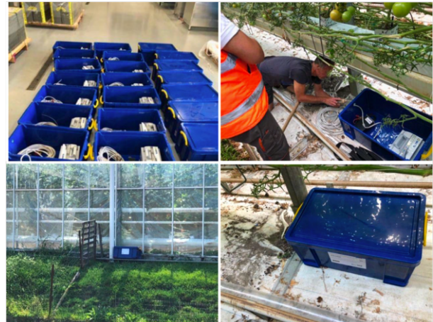
Figure 4: Installation of the seismic sensors that monitored the geothermal operation of Nature's Heat project in Kwintsheul, The Netherlands.
