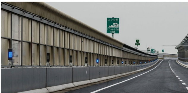
Fig. 1 Moving light guidance system at the Fukae Sag section on the Kobe Route of the Hanshin Expressway
