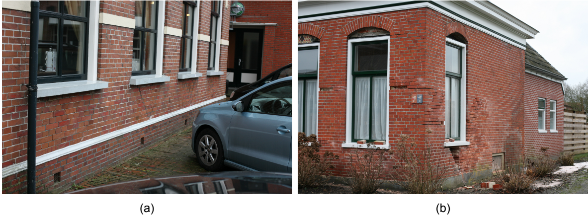
Figure 1.2: Damage on buildings in Groningen. (a) mortar failure, already filled cracks under the windows and (b) mortar failure, loose bricks are taken out. Photos by Harm Hoorn.
