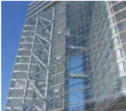
Figure 4.6: Stadttor Duesseldorf, Petzinka, Pink und Partner, 1998 Corridor façade: The outer pane (function: tightness and solar penetration) and the inner façade (function: wind tightness and room enclosure) are almost one metre apart.
