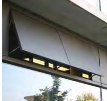
Figure 5.18: Weather-protected night ventilation flap installed below concrete projections
