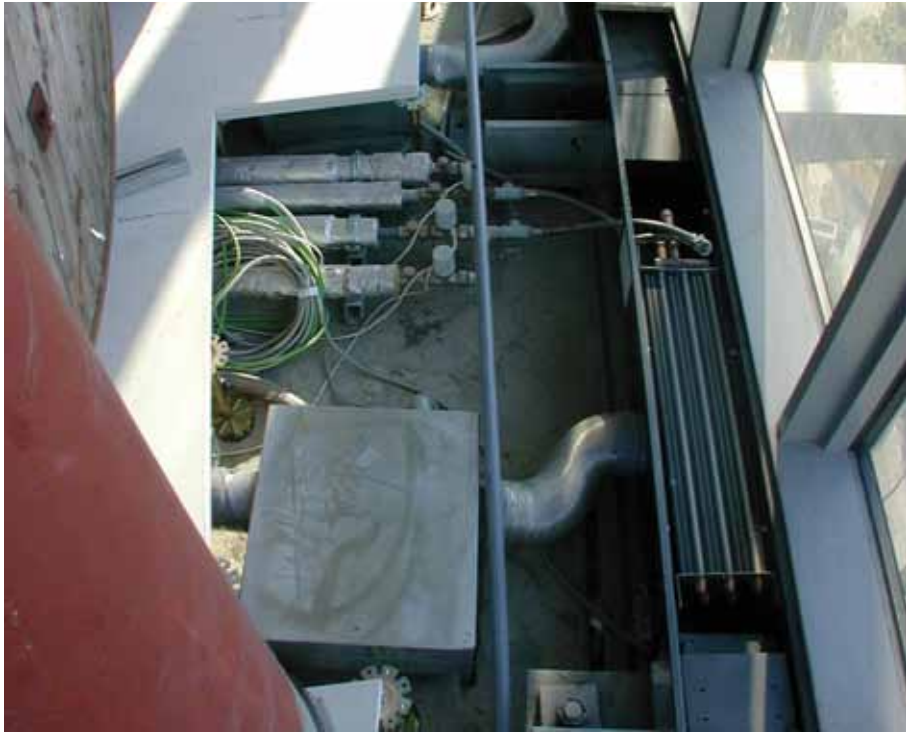
Figure 5.24 Decentralised ventilation components in a suspended floor; air and water supply lines are clearly visible
