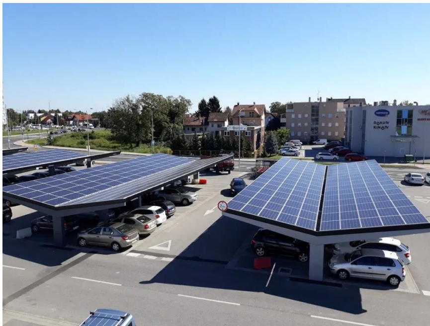
Figure 2.5: Example of installed solar carport [6]
