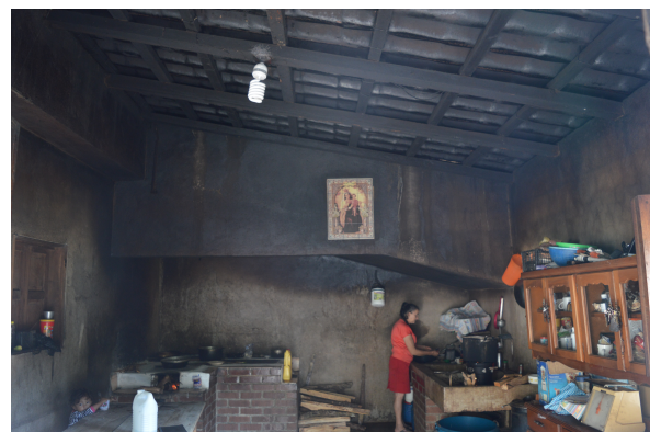
(b) A typical house with the roof and walls covered with emissions
