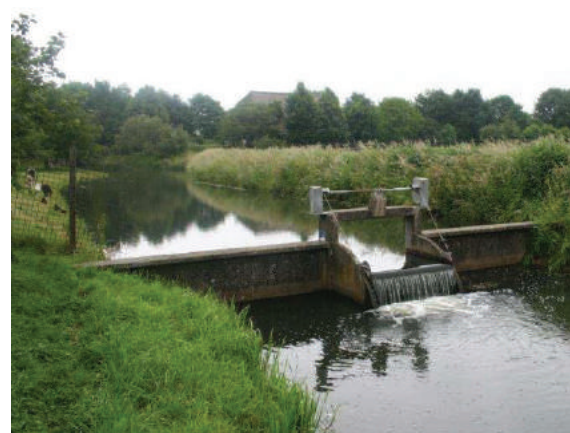
Fig. 80b: An example of an adjustable water structure for the salt water channel for the inlet of salt water (a dam)
