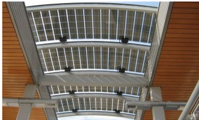
Figure 19: Example of curved glass solar panels used in the roof windows of a building (Movares, n.d.)
