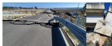
Figure 3. Abutment rotation due to soil liquefaction [18]
