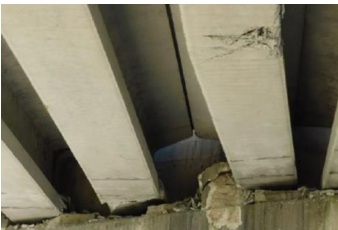
Figure 5. Lack of End Diaphragms [18]
