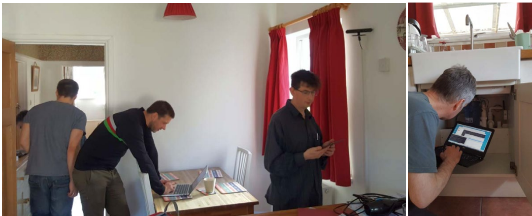
Figure 8 Pilot home installation
