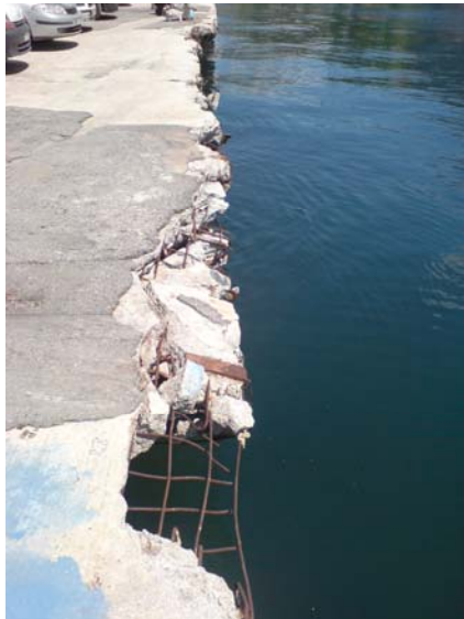
Figure 48 Severe deterioration at Quay 1 of the P.T.
