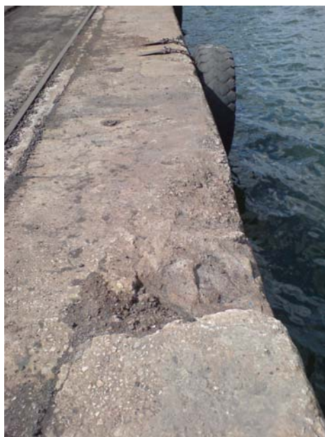
Figure 41 Cracks at Quay 20
