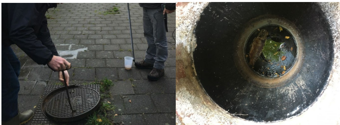
Figure SI 1.3 Example of a manhole of the groundwater drainage system (the dead fish indicates the possible back flow from the ditch to the drain manhole)
