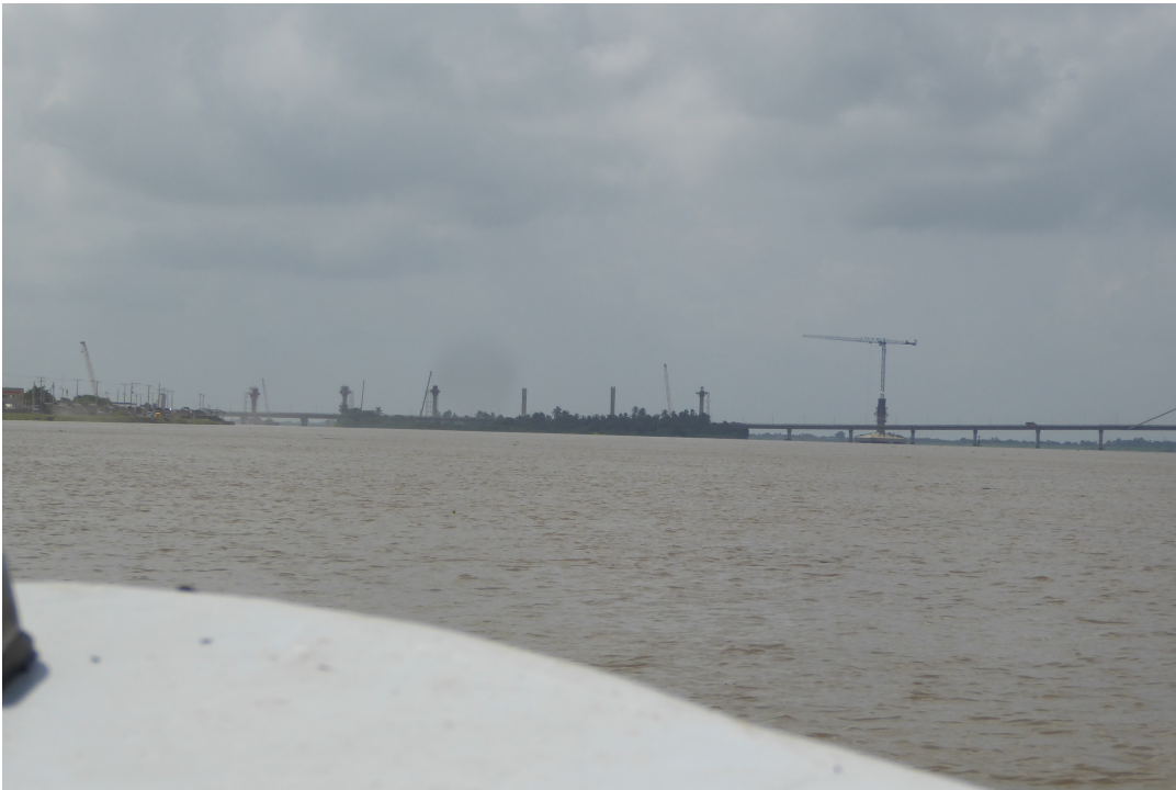
Figure K.3: Current Pumarejo bridge and construction of new Pumarejo bridge (September 20, 2017).
