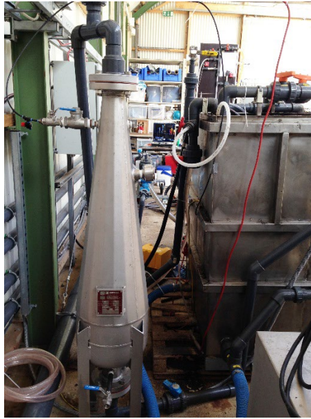
Figure 20 Speece cone at the Harnaschpolder WWTP, The Netherlands (source: C. M Barreto).
