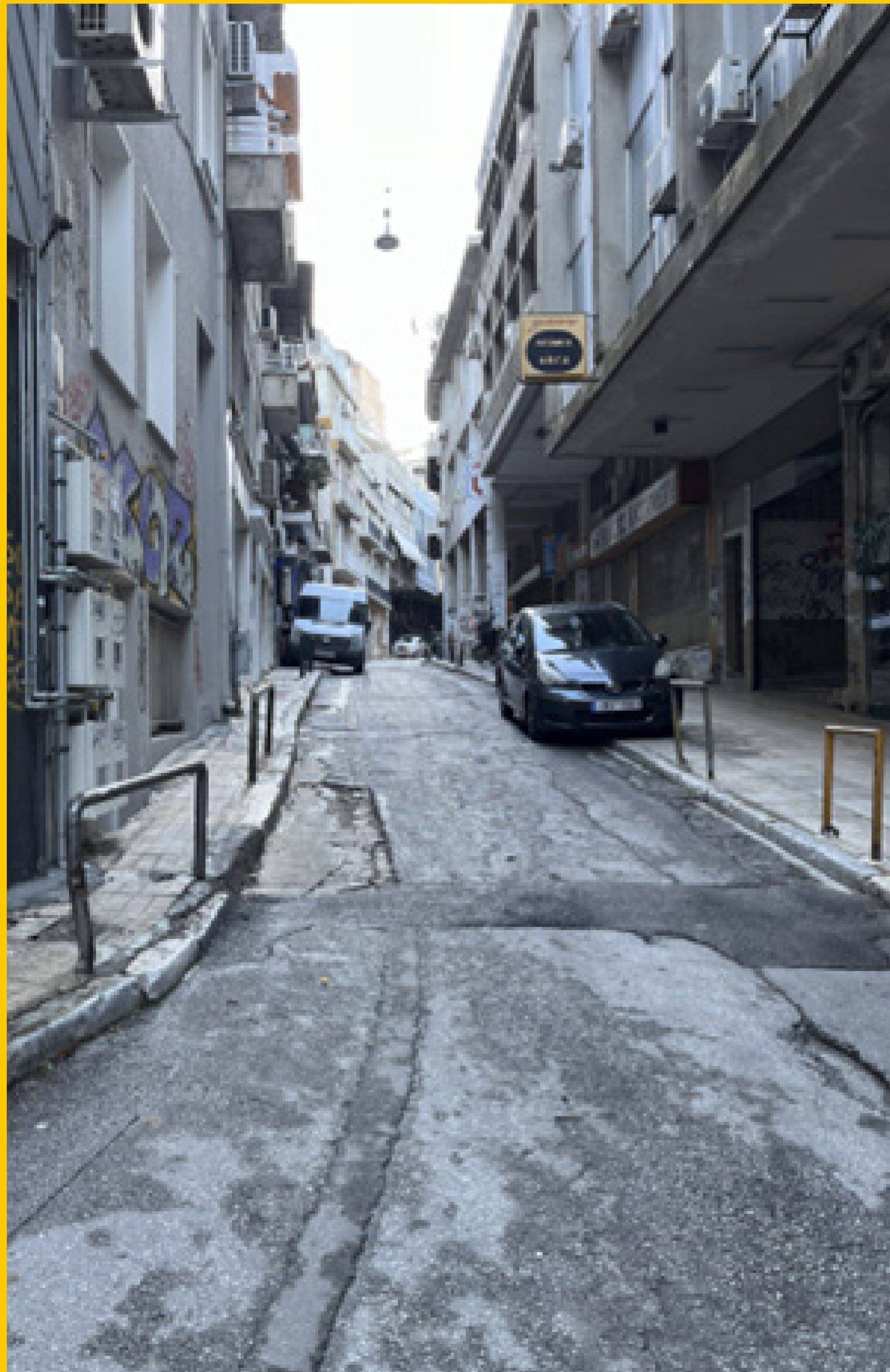
Figure 1.1 Minor infrastructure deterioration in Athens, demonstrating uneven asphalt patching and a bent sidewalk guardrail. (Photograph by author, 2025).
