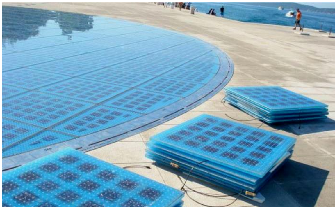
During construction the prefabricated panels with the PV cells and the LED lights. Also wires are needed ( http://hr.wikipedia.org/wiki/Pozdrav_Suncu )
