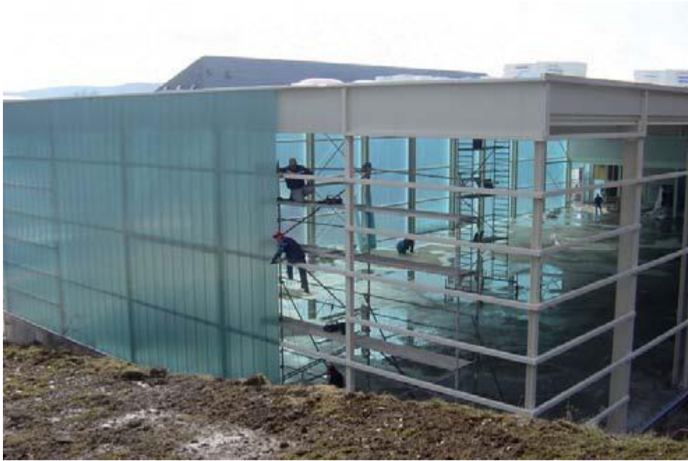
Image during assembling of the facade. Easy and quick installation with intermediate supports ( https://kluedo.ub.uni-kl.de/home )
