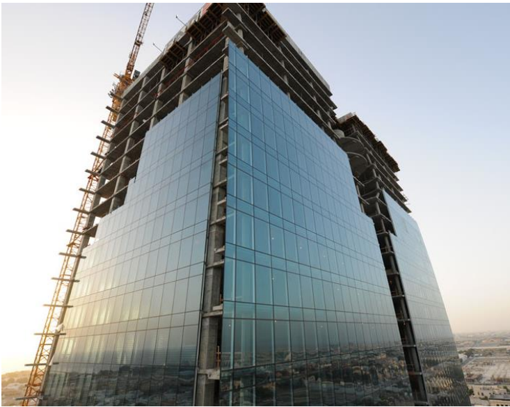
Image during the construction phase where the glass panels are mounted on the facade like a curtain wall system ( http://www.citiled.com/ )
