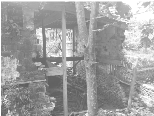
Image 5.4-2: Original sight of the valuable house in disrepair Source: Xiongliyue, sight of Tuochuan (2017).
