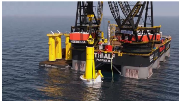
Figure 17. Image from simulation on how HMC will install the monopiles using a new designed template (HMC data, 2022).
