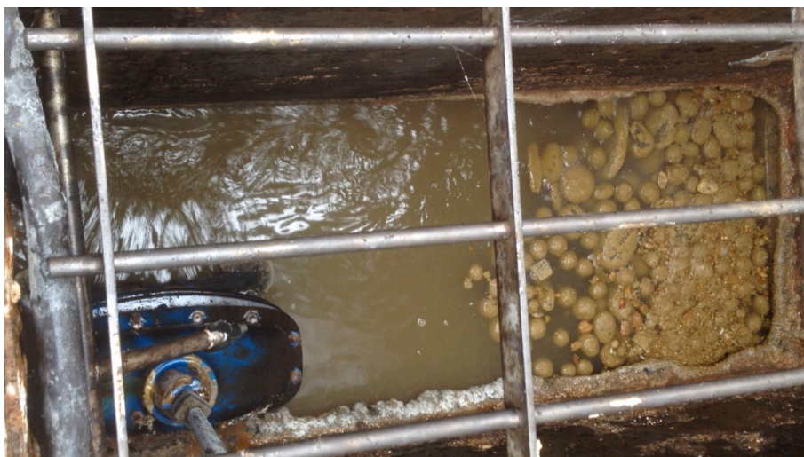
Figure 11 - FOG deposits in the small pumping station Millingenhof in Amsterdam, apparent as floating layers attached to the walls, floating balls and in bar shape.
