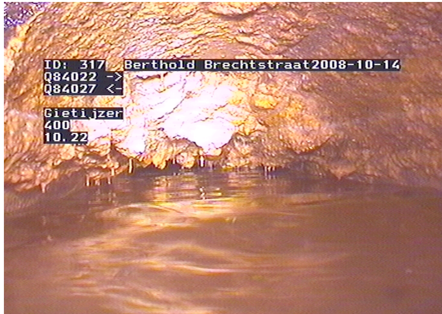
Figure 9 - FOG deposits in Amsterdam sewer pipes, located on the soffit (Source: Waternet)
