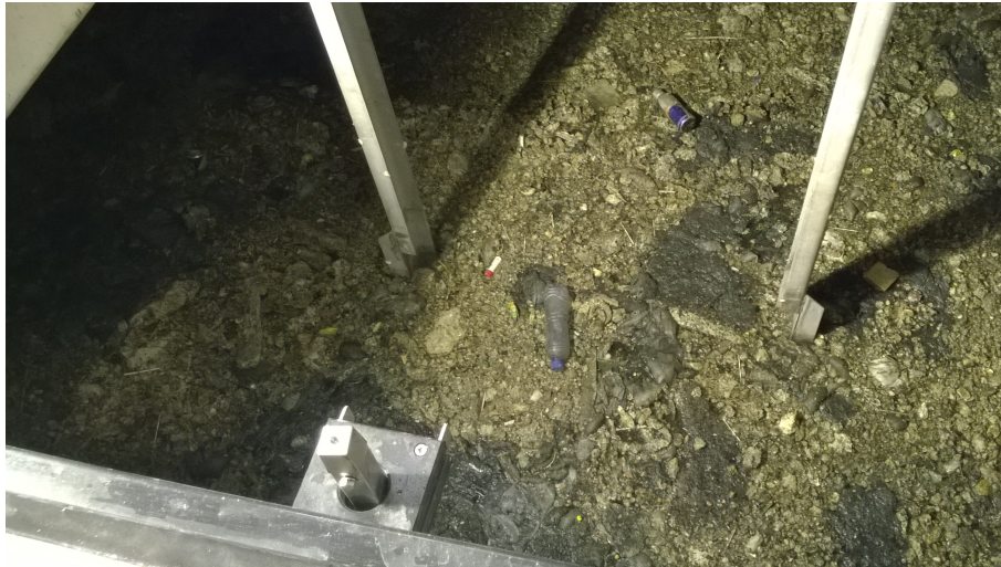
Figure 10 - Thick floating layer of FOG at the large pumping station Amelandseplein in Rotterdam (source: Municipality of Rotterdam)
