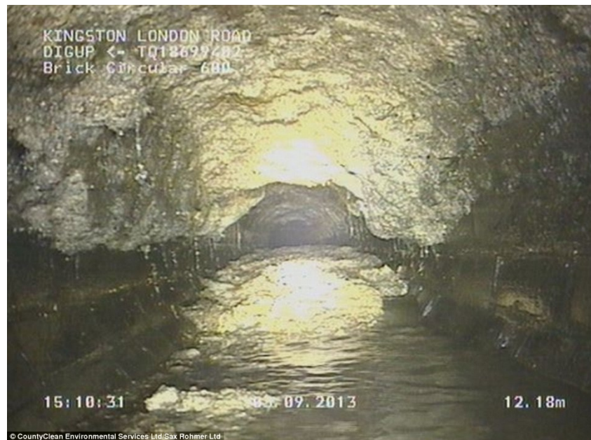
Figure 1 - Severe accumulation of FOG in London's sewer system (Glanfield, 2014)
