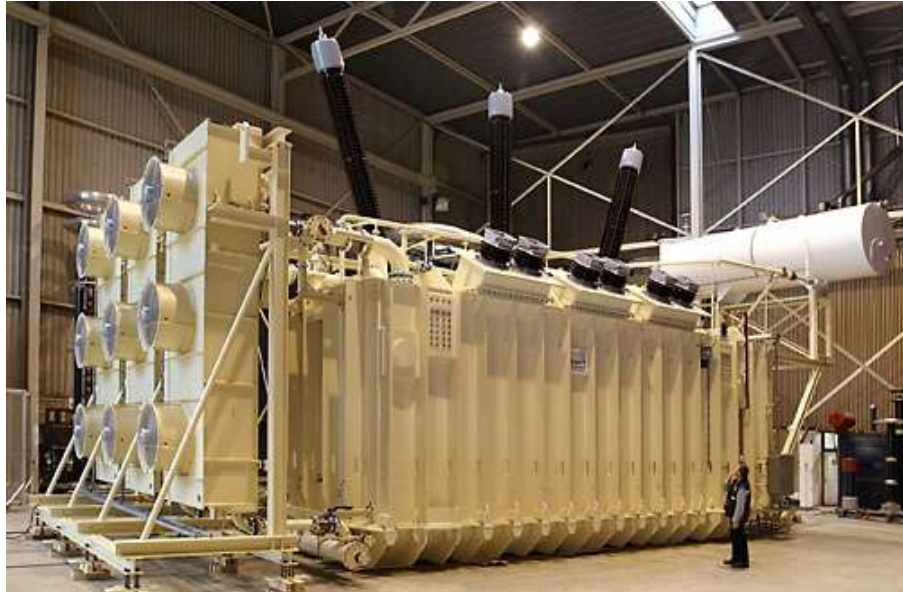
Figure 1-3: One of the large transformers manufactured by SMIT transformers, Nijmegen [1]
