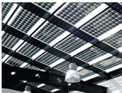
Skylights with BIPV
