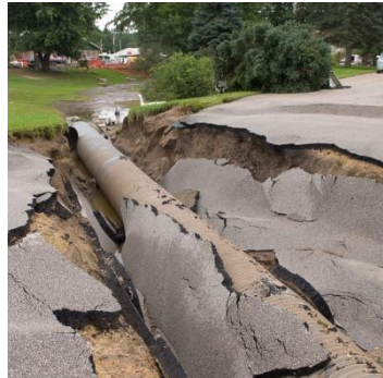
Erosion of culverts
