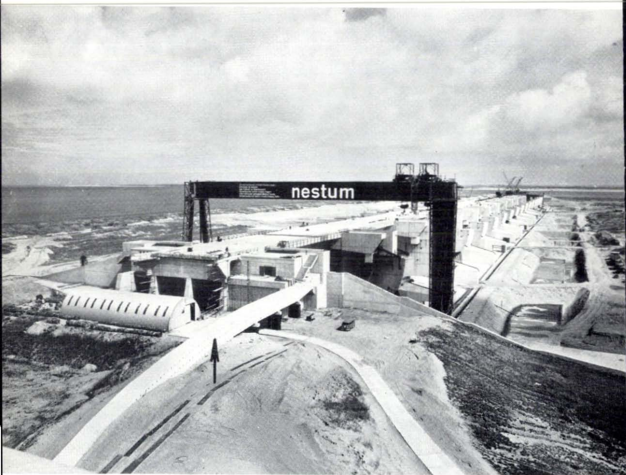
Figure 39. Nestum crane. In the foreground the duct (see arrow) for the electricity cables between control room and southern abutment
