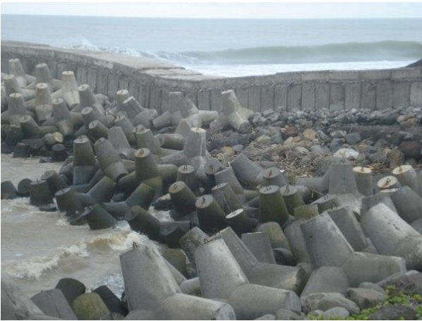
FIGURE 1-1 LOCAL FAILURE OF THE WESTERN BREAKWATER
