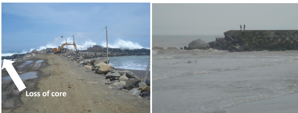
FIGURE H-6 LOSS OF CORE AND DAMAGE TO THE HEAD OF THE BREAKWATERS (PROF. NUR YUWONO, 2015)
