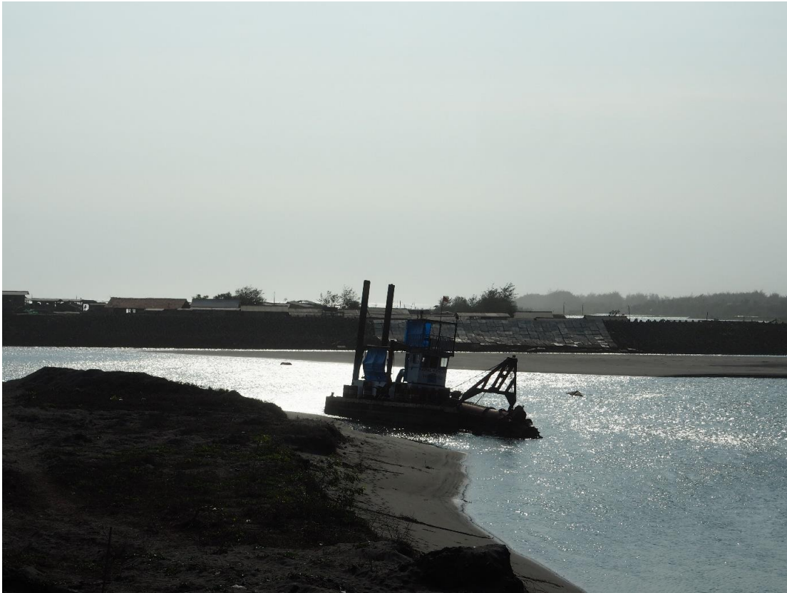
11. Dredging works seen from the eastern jetty. On this picture the large amount of sediments in the navigation channel can be seen. In the back the repair works from a ship collision can be seen.
