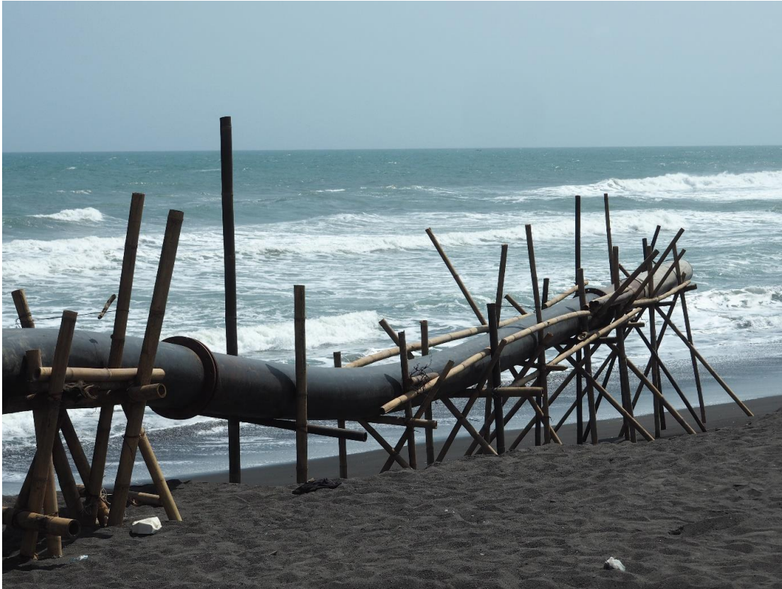
12. Tube which is used for the dredging works of the navigation channel.
