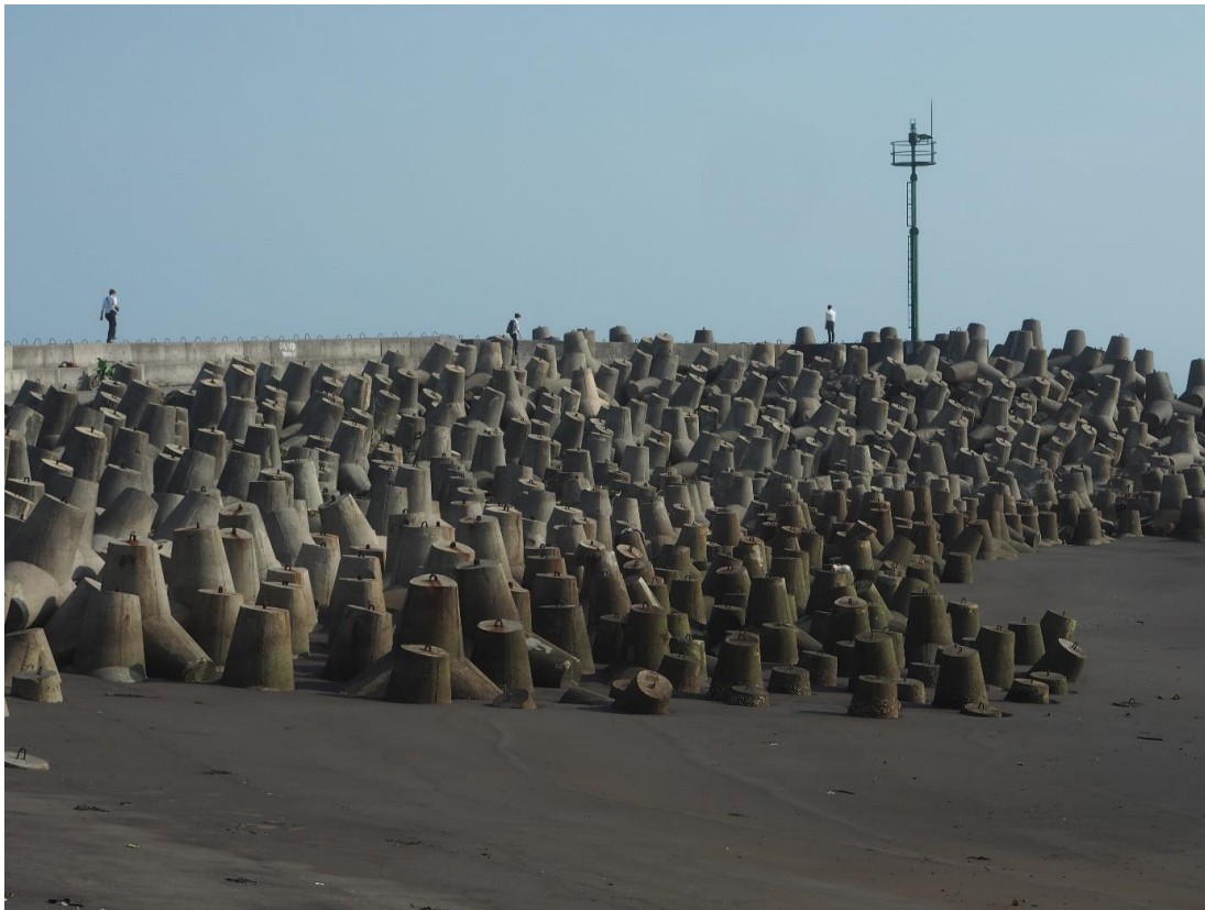
13. Large sedimentation on the inside of the jetty.
