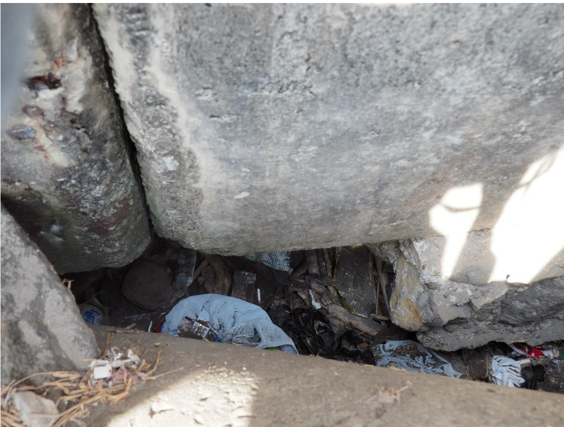
8. A gap below the concrete pavement.
