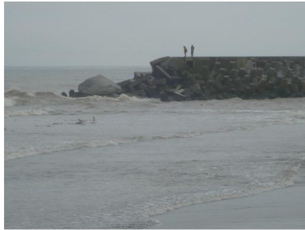
FIGURE 1-2 COLLAPSE OF THE TIP OF THE BREAKWATER
