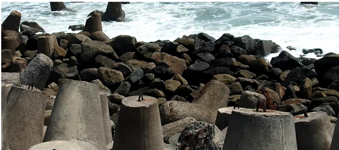
6. The core material is exposed to the waves because of the collapse during construction. There are no tetrapods placed on top of the core.
