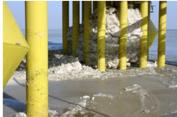
(b) Internal ice jam in between the conductors.
