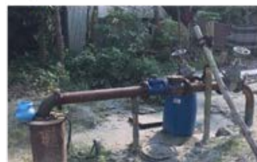
1, Main pipe supply and ground water pump
