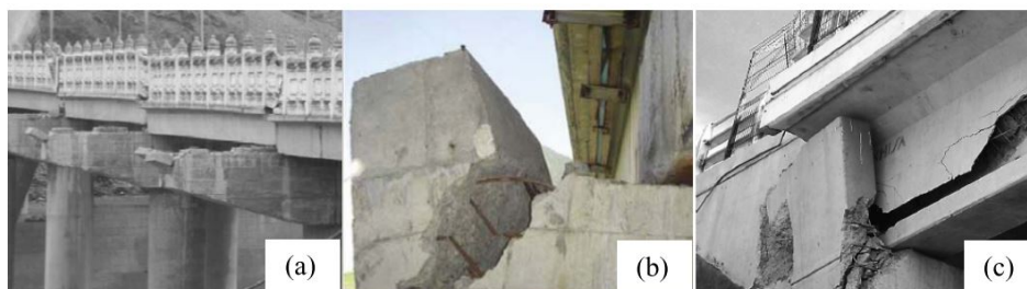
Figure 2.11. Typical shear key failure: (a) totally shear of; (b) diagonal shear failure; (c) flexural failure [Megally et al., 2002].
