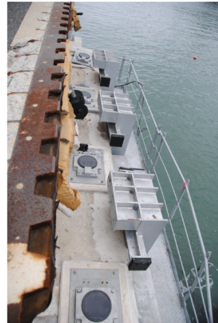
Figure 1.3. Bridge uplifted before lateral movement [Bricker and Nakayama, 2014].
