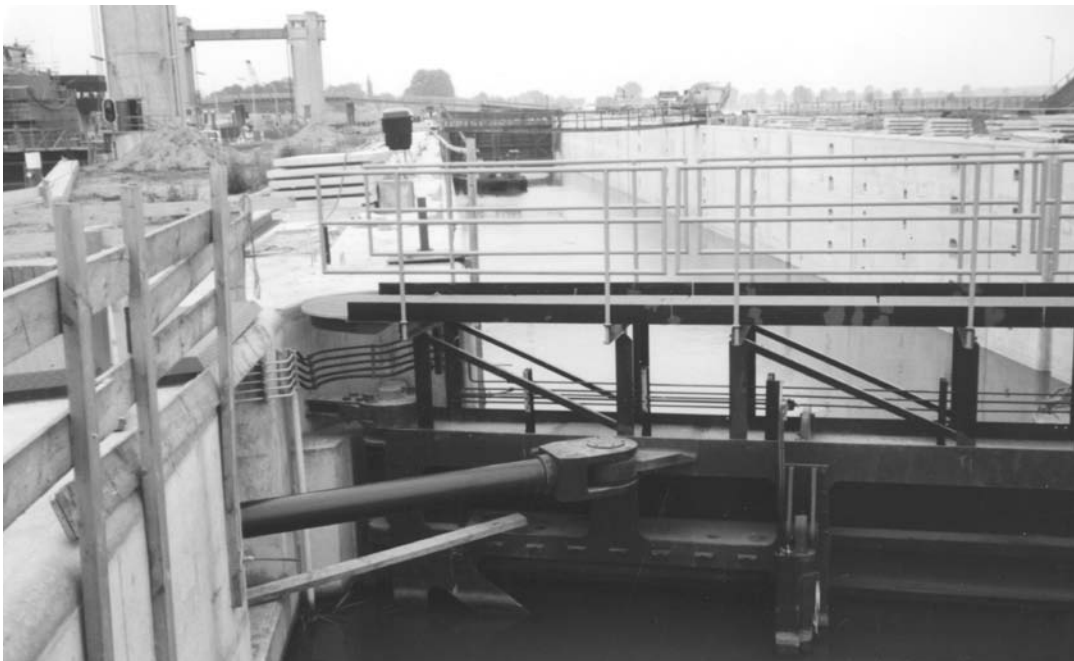
Photo 7.20 Hydraulic cylinder gate operating mechanisms of Tweede Sluis at Lith
