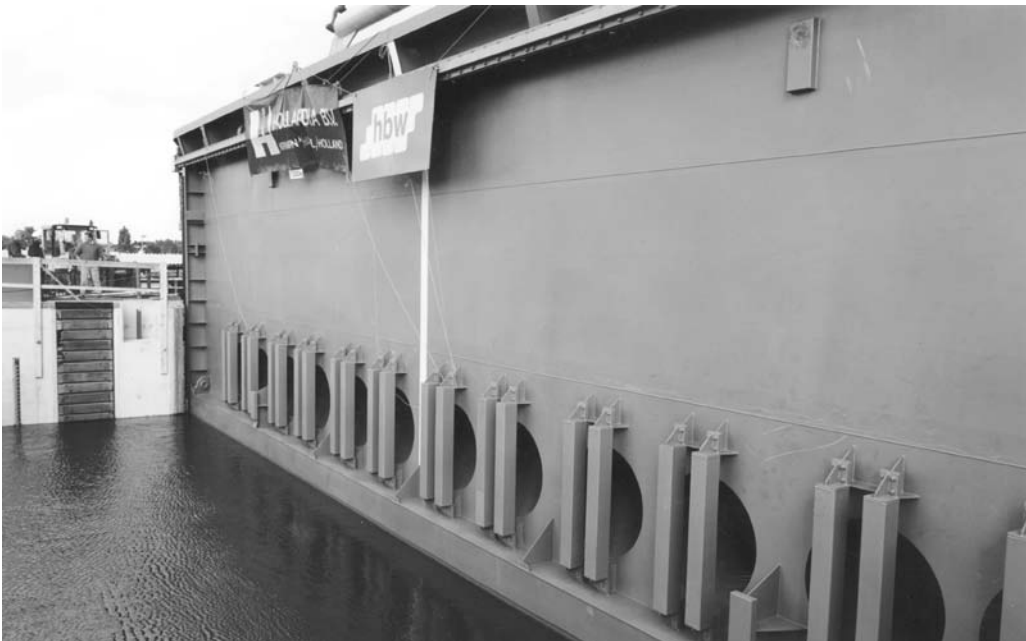
Photo 6.13 Energy dissipating bars behind the round openings of the sliding gate of Nieuwe Oranje lock in Amsterdam
