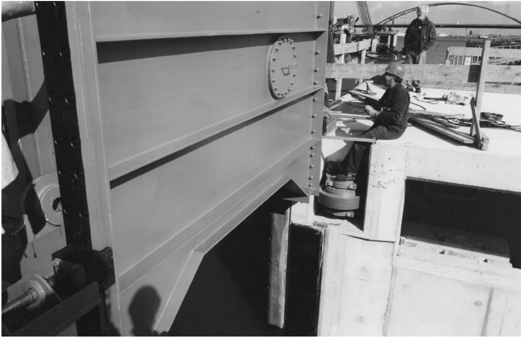
Photo 7.30 Horizontal guide wheel of the sliding gate at Nieuwe Oranjesluis in Amsterdam
