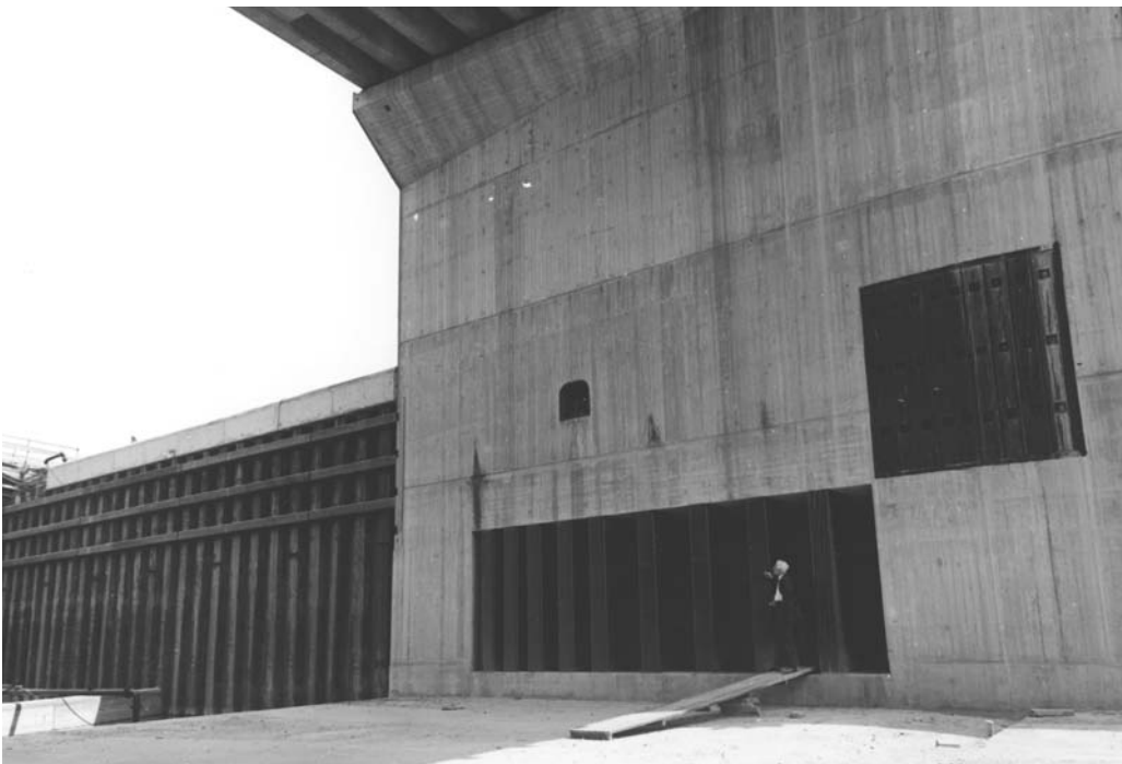
Photo 6.19 Outflow opening of the bypass culvert of the lower head of the locks at Maasbracht
