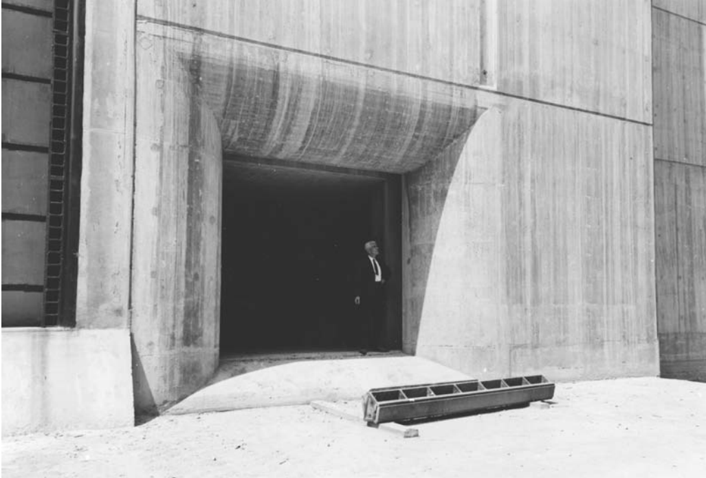
Photo 6.18 Inflow opening of the bypass culvert of the lower head of the locks at Maasbracht
