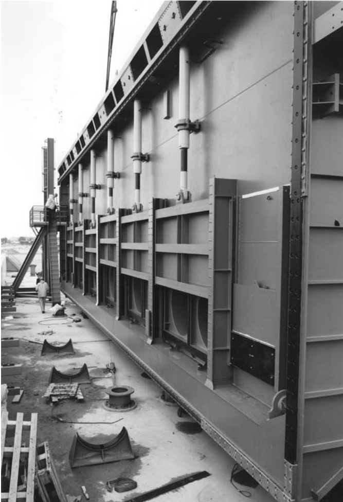
Photo 6.12 Sluice gates in front of the round openings of the sliding gate of Nieuwe Oranje lock in Amsterdam
