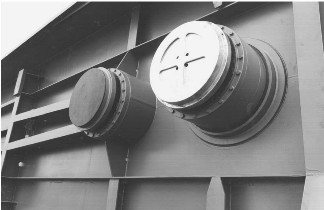
Photo 7.28 Fixed load bearing shoe and hydrostatic bearing of sliding gate of Nieuwe Oranjesluis in Amsterdam
