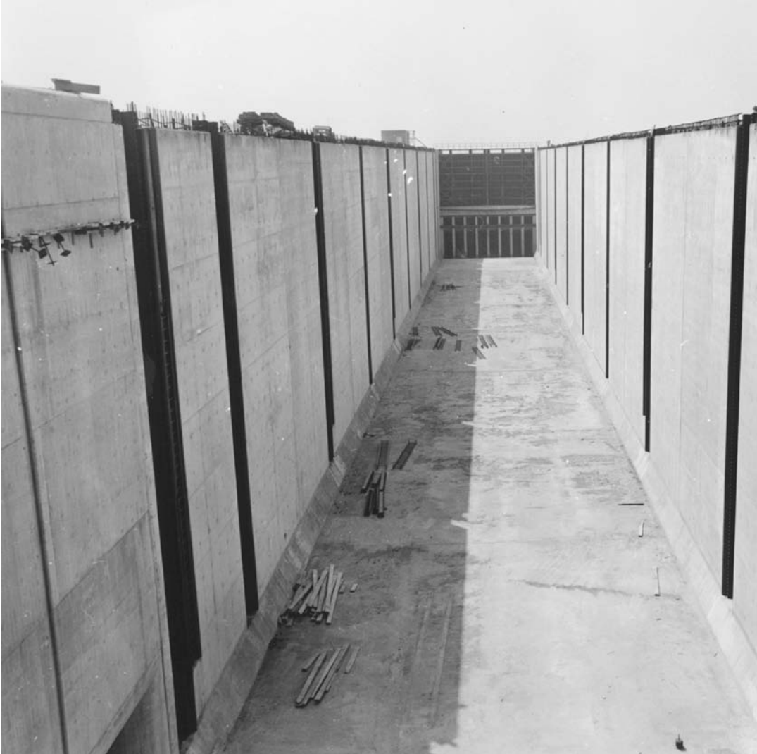
Photo 9.1 Lock chamber of the navigation locks at Maasbracht
