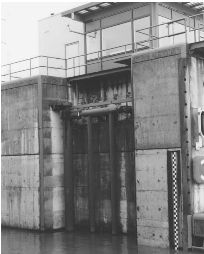
Photo 7.21 Frame shaped locking device for single pivot gate of the lock at Nieuwe Statenzijl
