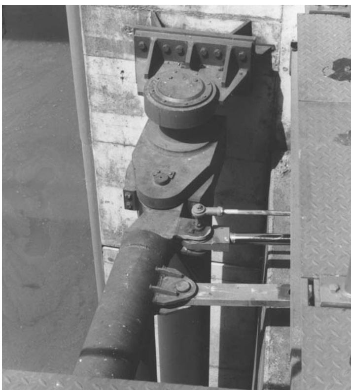
Photo 7.22 Detail of the locking device for single pivot gate of the lock at Nieuwe Statenzijl
