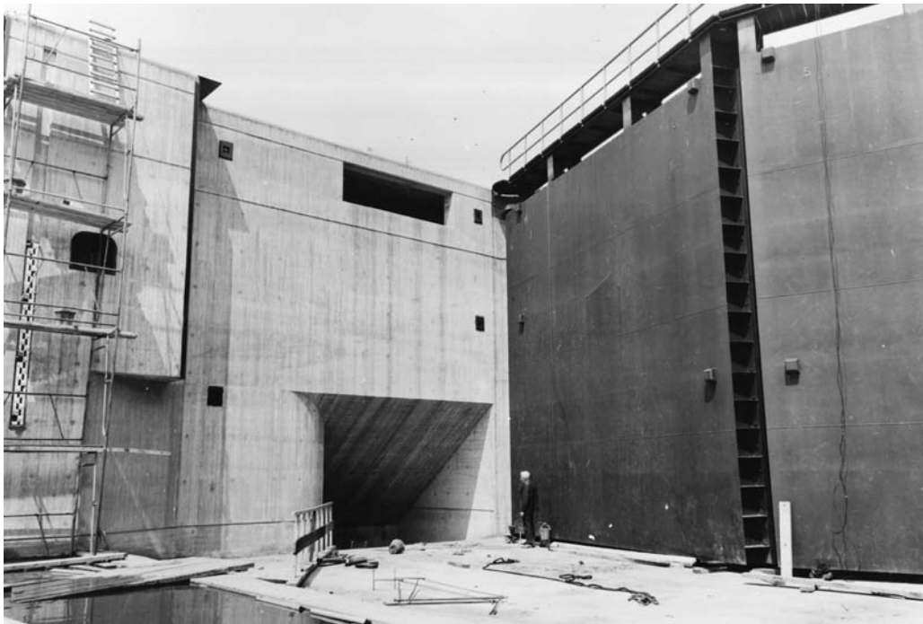
Photo 6.14 Inlet opening in upper head of the locks at Maasbracht
