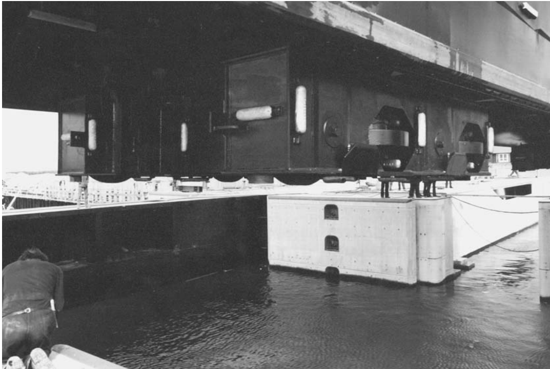
Photo 7.27 Lower roller carriage of the rolling gate at Middensluis in Terneuzen
