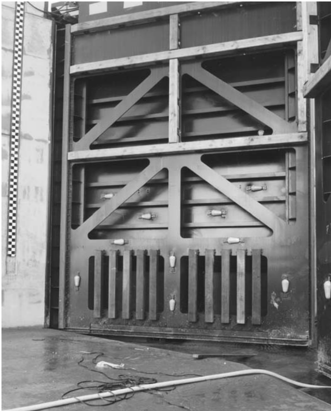
Photo 6.11 Energy dissipating bars behind the rectangular openings of the mitre gates of Kleine Sluis in IJmuiden
