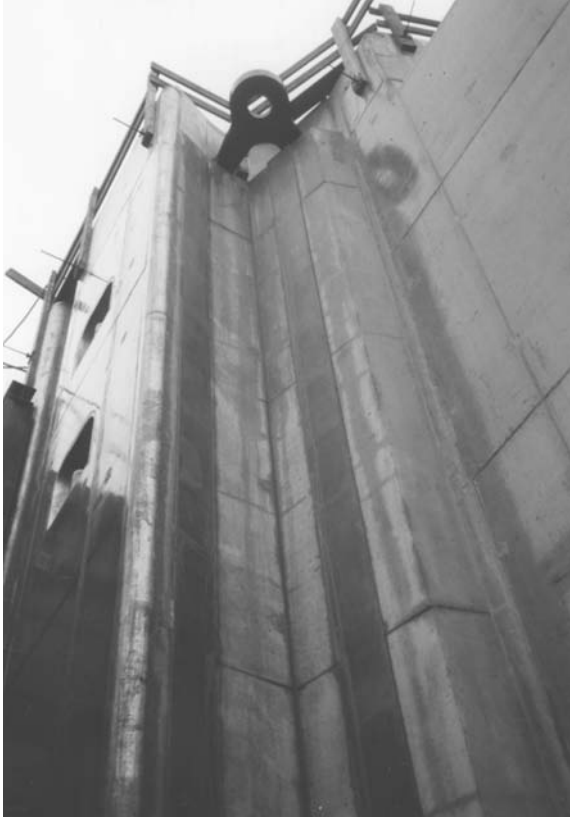
Photo 7.12 Support areas of the mitre gate at Tweede Sluis in Lith
