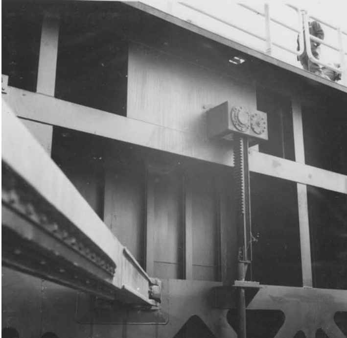
Photo 7.15 Direct rack bar for gate and sluice movement of Koopvaardersschutsluis in Den Helder
