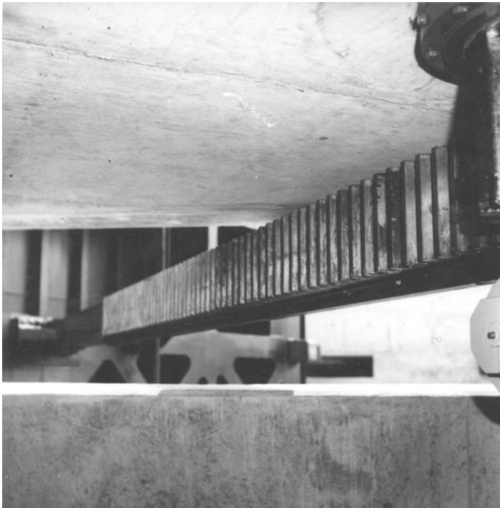
Photo 7.16 Direct rack bar for gate movement of Koopvaardersschutsluis in Den Helder
