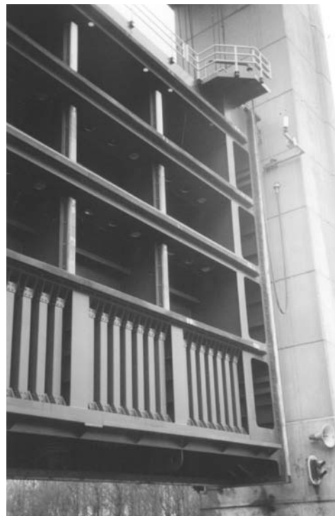
Photo 6.9 Energy dissipating bars behind the rectangular openings in the lift gates of the new locks in Weurt
