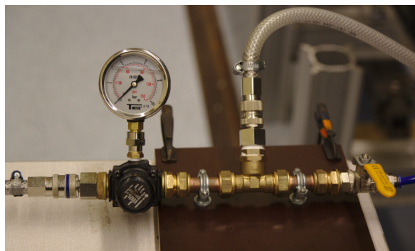
(b) Air supply and seeding controller - located outside of ST-15
