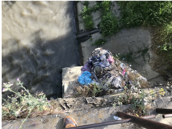
Figure 3.2: Garbage on bridge after flooding event
