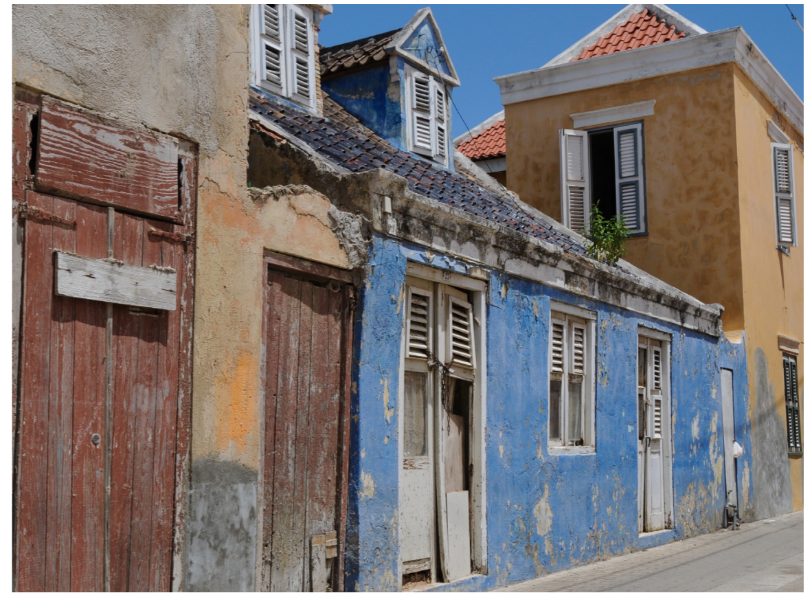
Dilapidated city houses in Otrobanda
