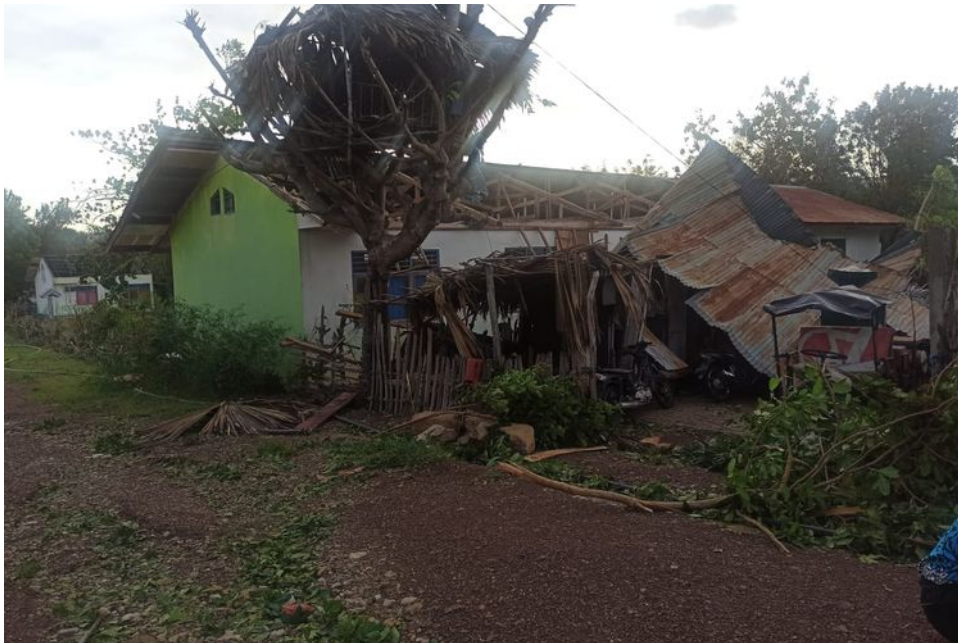
Figure 50. One example of a house for an operational laborer affected by the tropical cyclone Seroja (courtesy of UPP Class III Port of Seba)
