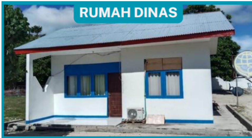
Figure 49. The condition of the Ministry of Transportation Official Residences near the Port of Seba after tropical cyclone Seroja (Courtesy of Ministry of Transportation)
