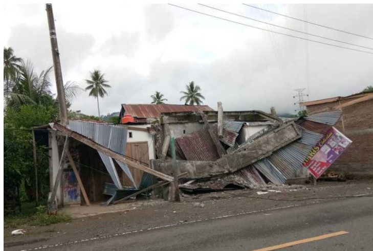
Figure 65. The condition of residential houses around Mamuju Simboro Port was affected by the earthquake, and some of the residents are employees of the port.
