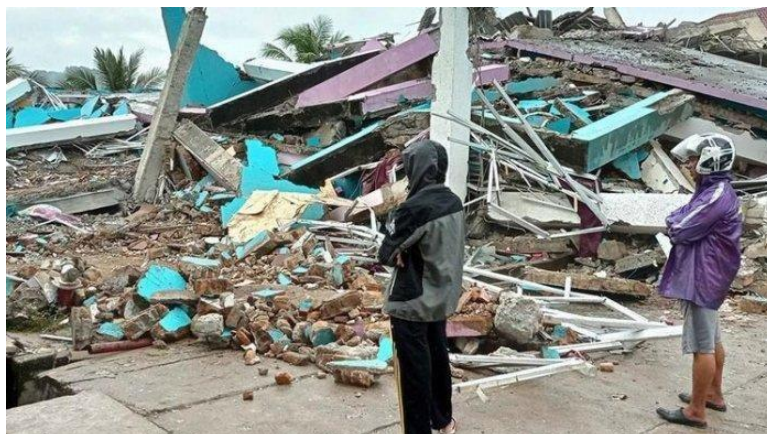
Figure 66. The condition of several officer housing units at the Port of Mamuju Simboro following the Majene aftershock on the early morning of January 15, 2021.
