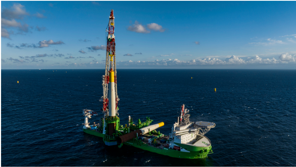
Figure 3.1: Orion of DEME installing monopiles with a diameter of 9.5 metres at Arcadis Ost in June 2022 [42]
